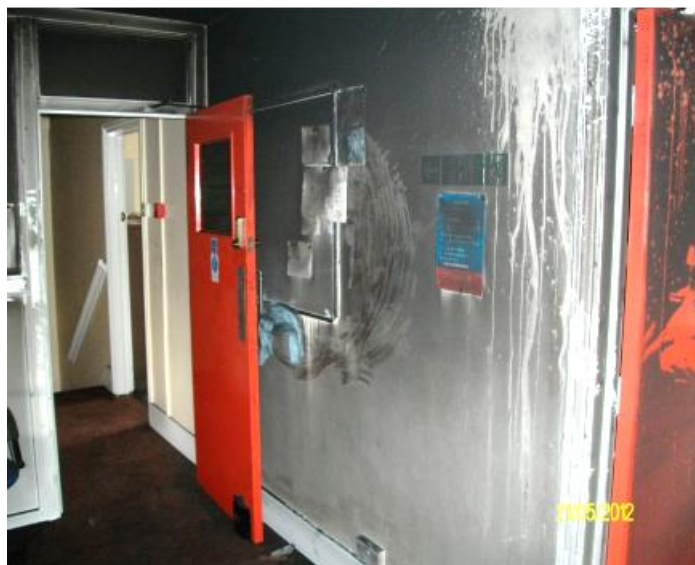
This fire door (closed at the time of fire) has held back the passage of heat and smoke. The room to the right was the fire room and the door had been wedged open!
